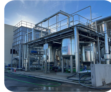
Thermal Hydrolysis Processing
