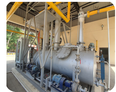
H 2 S Scrubbers
