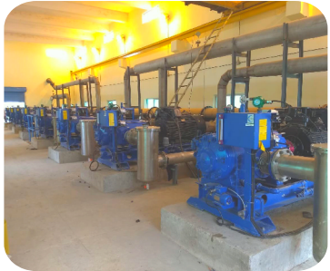
Biogas Recirculation Compressors
